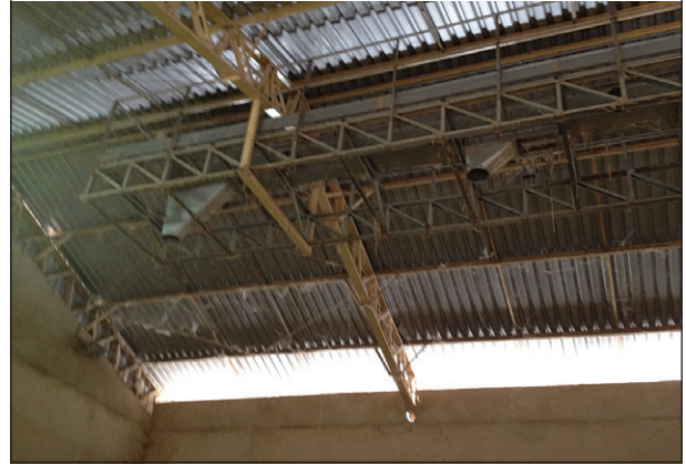
FIGURE 8 Openings in the ceiling allow the entry of pests, birds and dust that can contaminate the production environment
